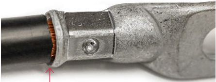
Figure 6, Gap between the terminal and insulation of the conductor.
